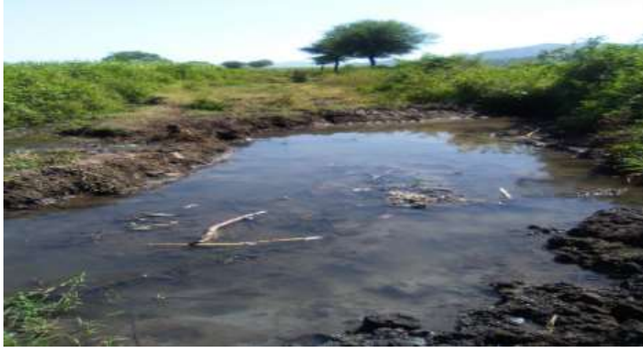
Figure 5. Silt deposition in tertiary canal.
